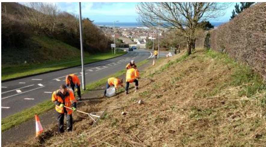
Northam Special Verge – the pavement and mown verge create a safe gap between the volunteers and the carriageway.
